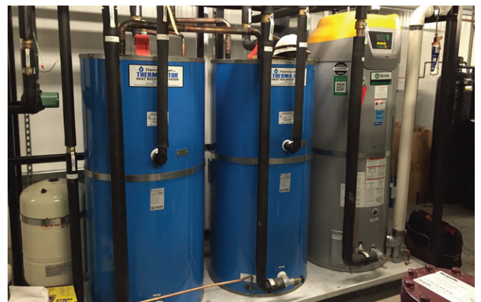
The refrigeration system uses the reclaim heat benefit from using Solstice N40.
