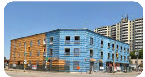
Closed-cell spray foam is being applied over the membrane on the exterior walls to meet Passive House requirements.
